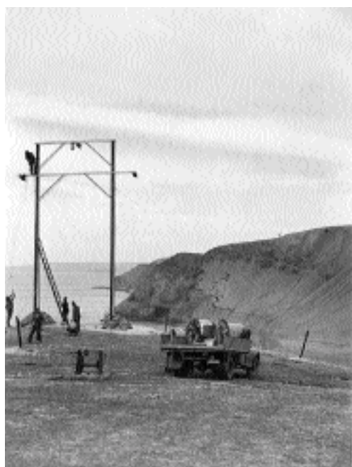
AESCo, AS PART OF THE WAR EFFORT, EXTENDED TRANSMISSION LINES TO PLACES LIKE BHP’S RAPID BAY QUARRIES. SHOWN HERE IS THE LINE BEFORE IT DESCENDS TO THE QUARRY AND SUBSTATION ETSA MUSEUM
