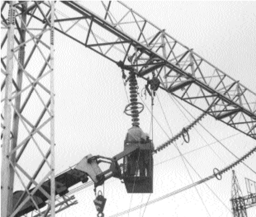
THE BEGINNING OF THE INTERCONNECTION PROJECT – WORKING WITH TRIPLE CONDUCTORS AT THE TALEM BEND SUBSTATION, 1983 ELECTRA NET SA
