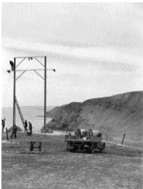
AESCo, AS PART OF THE WAR EFFORT, EXTENDED TRANSMISSION LINES TO PLACES LIKE BHP’S RAPID BAY QUARRIES. SHOWN HERE IS THE LINE BEFORE IT DESCENDS TO THE QUARRY AND SUBSTATION ETSA MUSEUM
