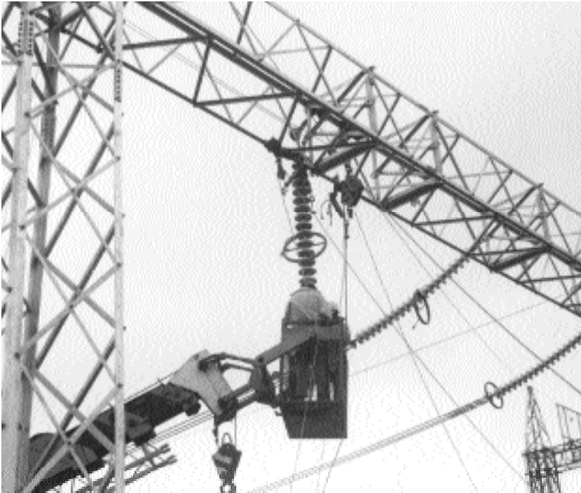
THE BEGINNING OF THE INTERCONNECTION PROJECT – WORKING WITH TRIPLE CONDUCTORS AT THE TAILEM BEND SUBSTATION, 1983 ELECTRANET SA
