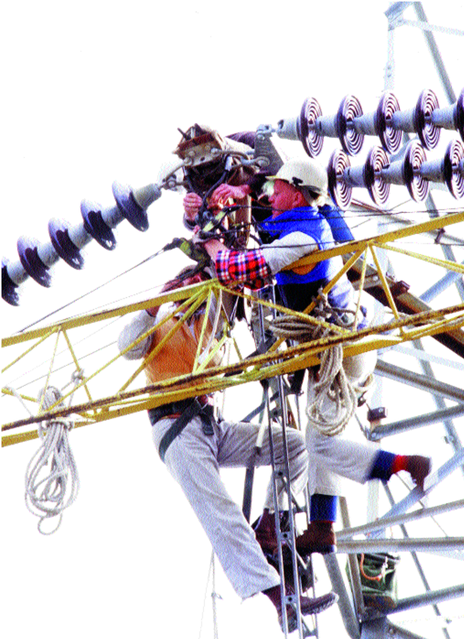
PAGES 68,69 AND 70: TRANSMISSION CREWS AT WORK – THEIR SKILLS ENTAIL USING STATE-OF-THE-ART EQUIPMENT AND TECHNIQUES ELECTRANET SA
